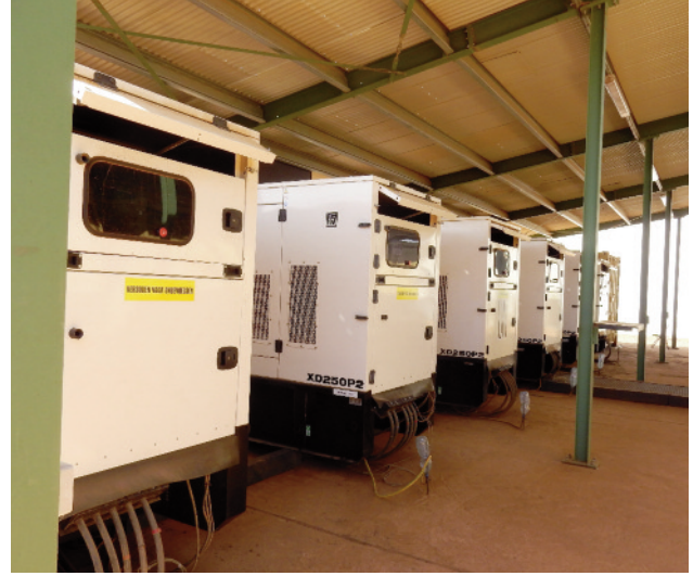
Photo 2. Hybrid energy plant at Camp Castor, Gao, Mali, 2016. Malkit Shoshan/FAST.
